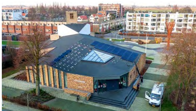
Figure 11: Image of modern church during installation of solar panels in the Netherlands as reported by De Roerom to illustrate a 2021 report by Radboud University .
