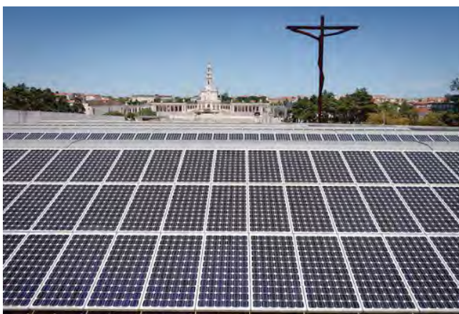
Figure 12: Solar panels installed on top of the Basilica of the Holy Trinity, overlooking the Basilica of Our Lady of the Rosary of Fatima used as an illustration in a report of Laudato Si' research in Portugal .
