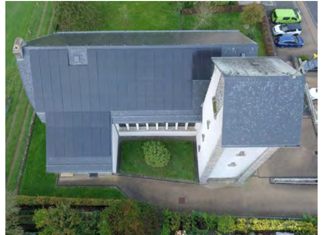
Figure 9: Church with '92 high-performance solar modules that has an annual energy yield of approx. 28,000 KWh' in Luxembourg as reported by the Archdiocese .
